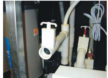
Spa Section Drain (Fig N)
