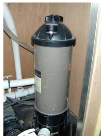
Picture of the filter column in the equipment bay
