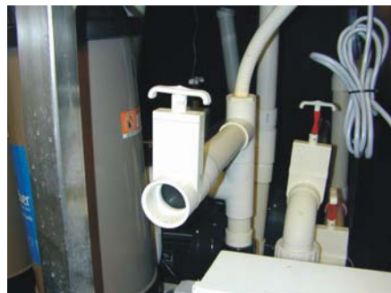
Spa Section Drain (Fig N)
